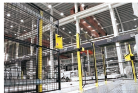
Safety light curtain
